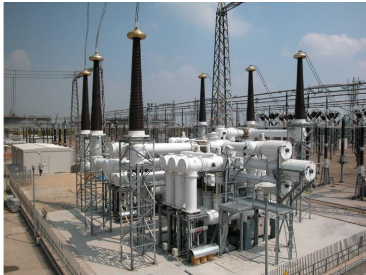
High voltage switchgear
